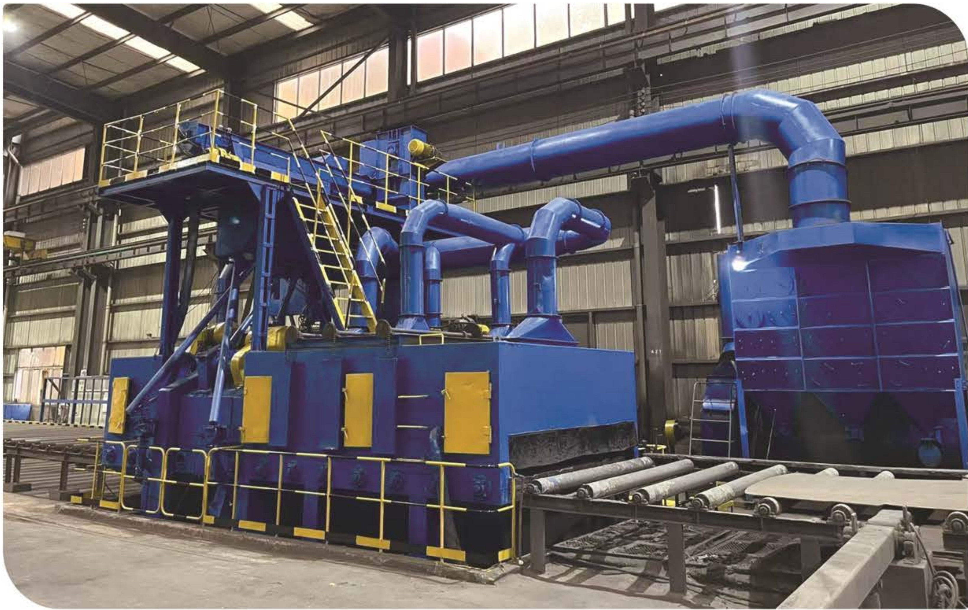
■ Steel pretreatment shot blasting machine
